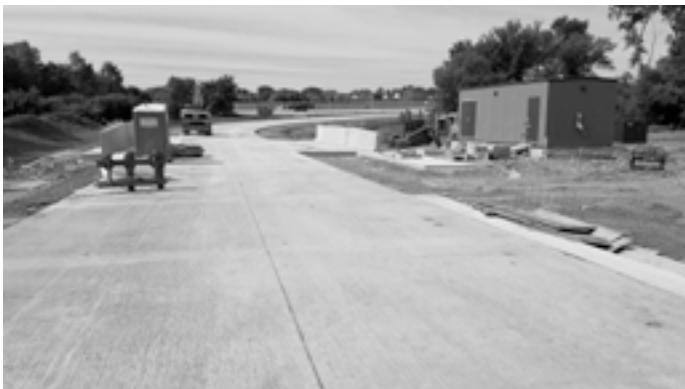
Figure 10. The improvements to the Central Road corridor include a new on-ramp to westbound I-90/Jane Addams Memorial Tollway which completes the full interchange at the I-90/Roselle Road complex.
