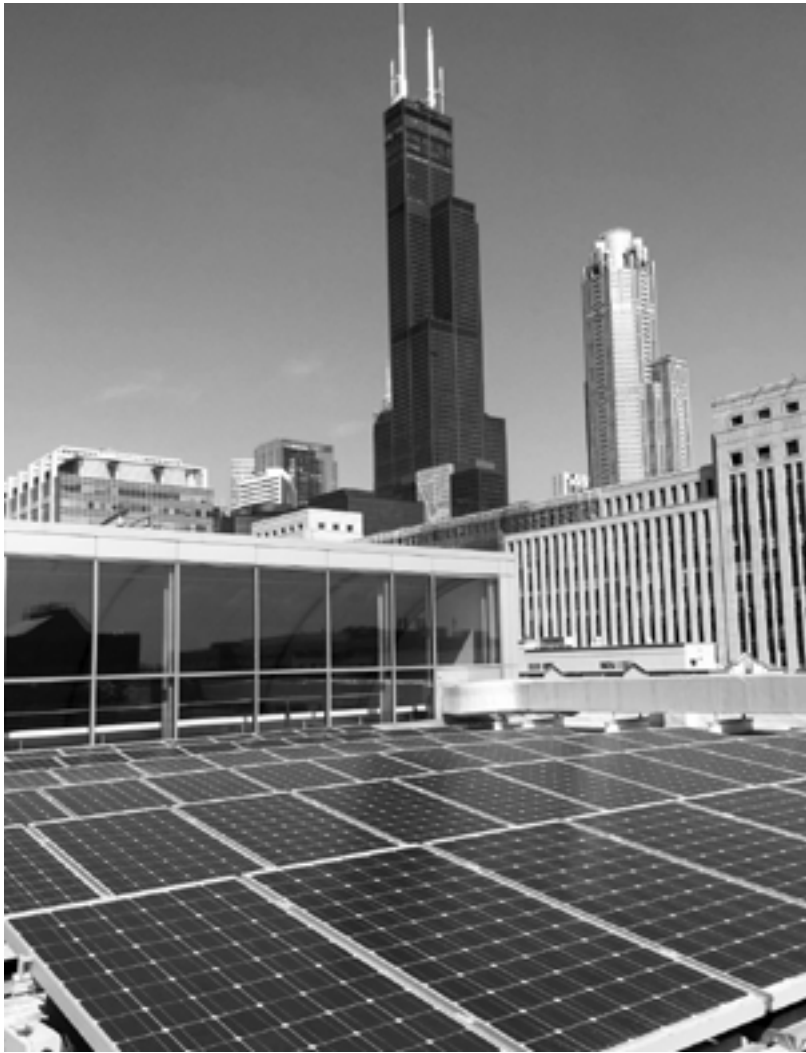
Domestic Violence Courthouse – Photovoltaic/Solar Panel Array
